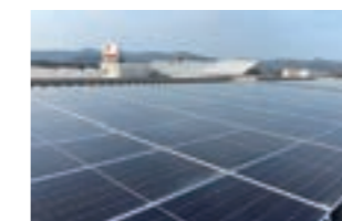
We have installed solar panels at the Kozakai and Ibaraki plants, which began generating electricity in April 2021.
